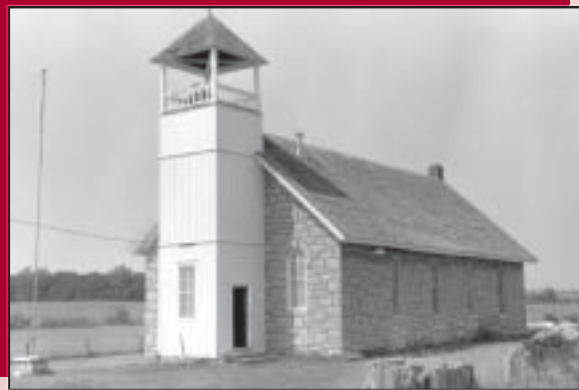
The long-term lessees of the Buck Creek School in Jefferson County are applying for state tax credits to offset some of the expense of lead paint removal.
