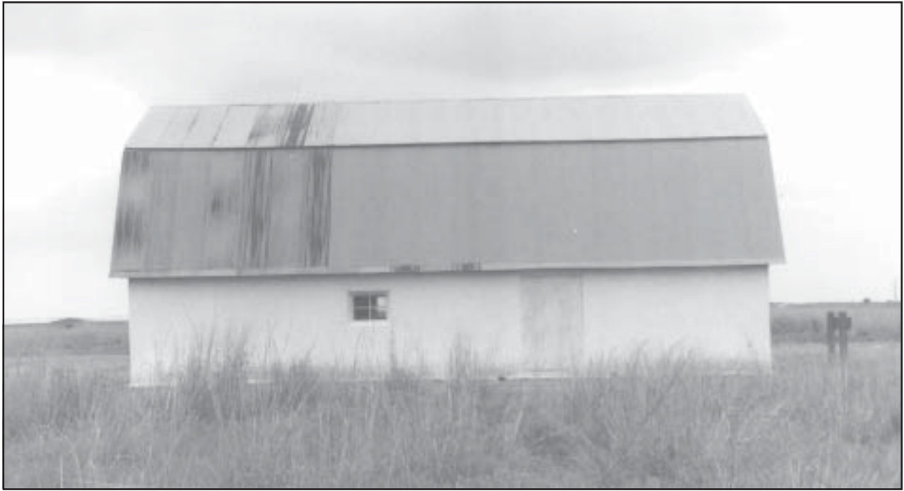
(Left and above) The Thornton Adobe Barn is an adobe dairy barn with a corrugated metal-clad gambrel roof. The walls of the lower story are constructed of adobe bricks covered on both the interior and the exterior with white stucco; the exterior walls of the hayloft are reused corrugated metal. A recent restoration effort has preserved the barn's unique adobe walls and rendered the barn weather-tight once again.
