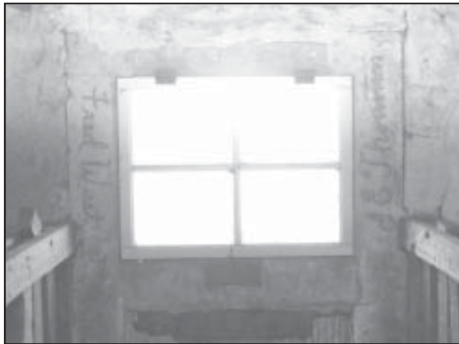
The pre-cast window casing on the west-facing wall is inscribed "Aug. 1942," while the casing in the north-facing wall is inscribed with the names of both Ed Thornton and Fred Westphal, a teenager who assisted Thornton in the construction of the barn.
